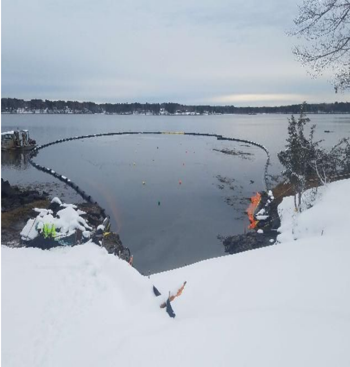
Fig 9: Turbidity curtain in place on west side of the Bay. Viewing east. (12-04-19).
