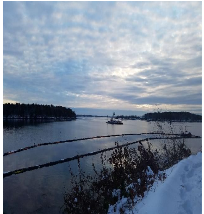
Fig 10: Mackworth installing turbidity curtain at Gundalow landing/east side of the Bay. Viewing west. (12-04-19).
